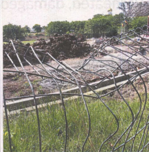
The stadium is in need of repairs and this includes its track, field and amenities as well as fencing.
