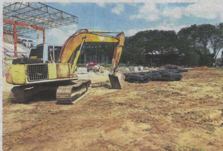
Ongoing earthworks at Stadium Sultan Suleiman are expected to continue until February next year.
